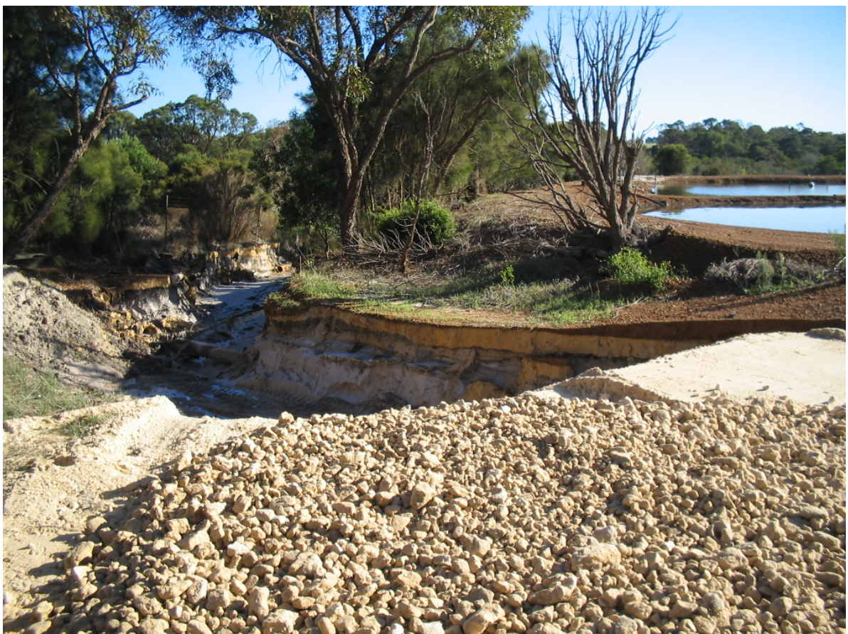
Photo 2 Damage to roadway at the Timewell Road WWTP following extreme rainfall, April 2004
