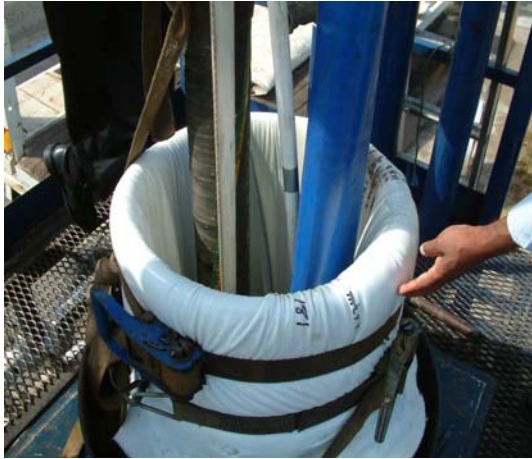
Trenchless Technology: This flexible liner is fed through a platform which stands over a sewer access chamber.
