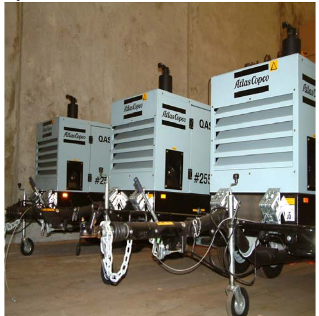
Ready for action: Mobile generators can be easily transported to site when required.
