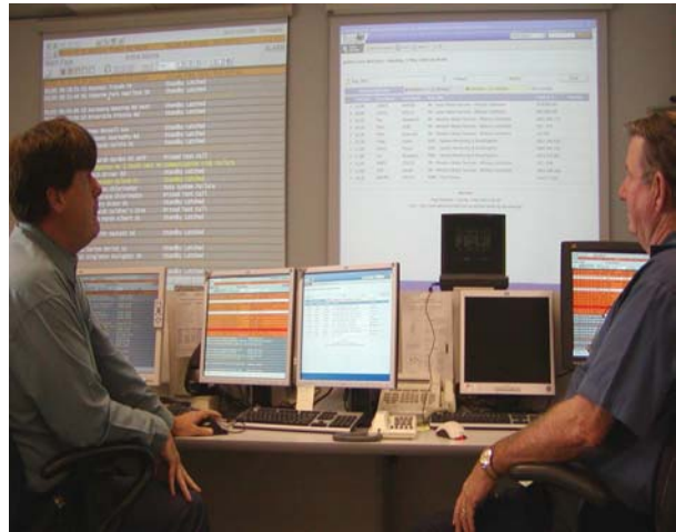
The Corporation electronically monitors its water and wastewater schemes 24 hours a day through the state-of-the-art SCADA monitoring system.
