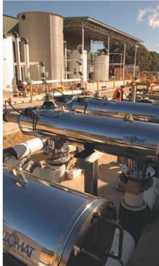
Advanced Water Recycling Plant
